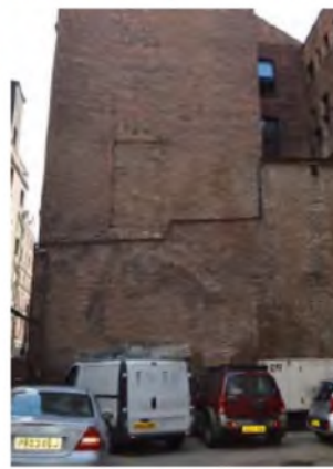
finlays warehouse adjacent wall
